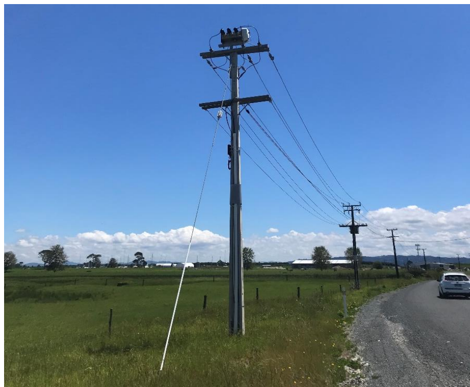
Figure 2: Overhead Reticulation comprising of; Pole Structure, Overhead Switchgear, Stay Wire and 11,000V and 400V Conductors.
