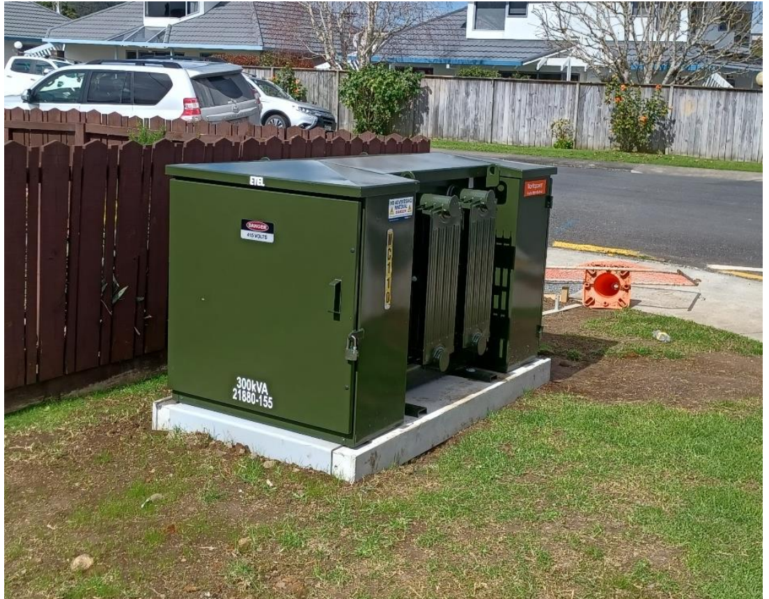
Figure 5: Underground Reticulation, Ground Mounted Transformer
