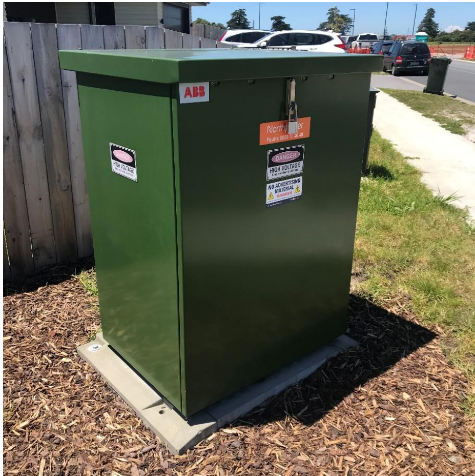
Figure 4: Underground Reticulation, Ground Mounted Switchgear
