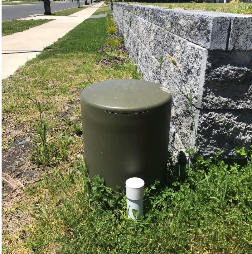
Figure 3: Underground Reticulation Standard Service Pillar
