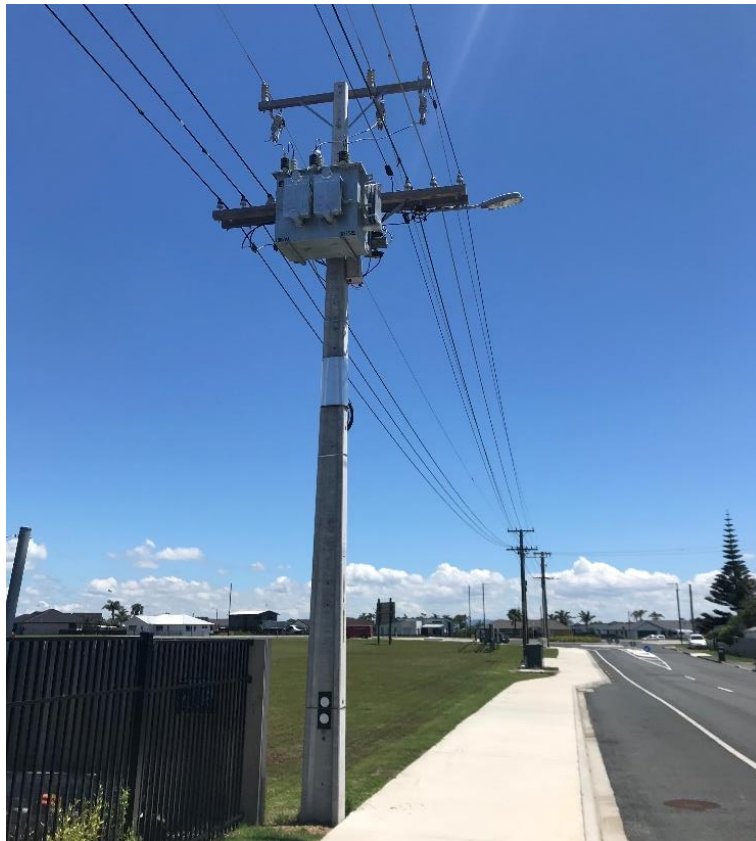
Figure 1: Overhead Reticulation comprising of; Pole structure, Overhead Transformer and 11,000V and 400V Conductors.
